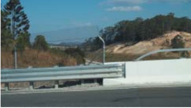
The bridge at Environ Road, Yelgun to Chinderah, shows a simple resolution maintaining constant height between road and bridge barriers.
