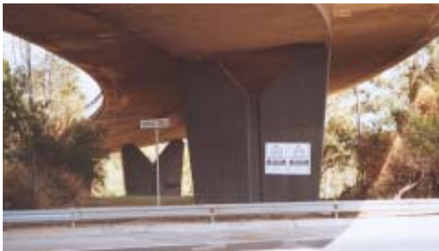
Deep overhang and acute angle of deck on this bridge on Victoria Road at Huntley's Point.
