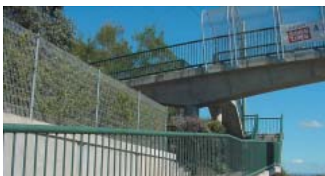
Complex and poorly considered stairs and walls.
