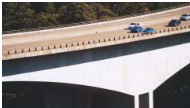
The twin bridges over the Mooney Mooney Creek employ a two rail parapet which optimises views of the landscape.
