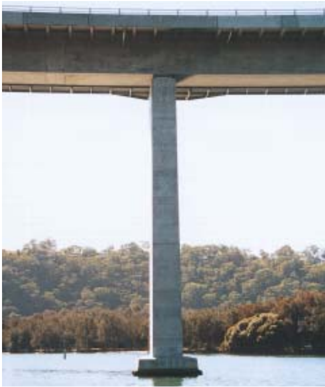
The piers of the bridge over the Woronora River have a slight taper of 1:100 sufficient to demonstrate refinement economy and elegance.
