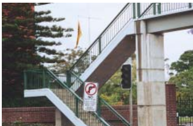
Where space is limited, stairs should be simple and compact as on this bridge over the Pacific Highway. Note the neat detail of the connection between superstructure and ramp marred only by staining. The handrail could have been a lot simpler.
