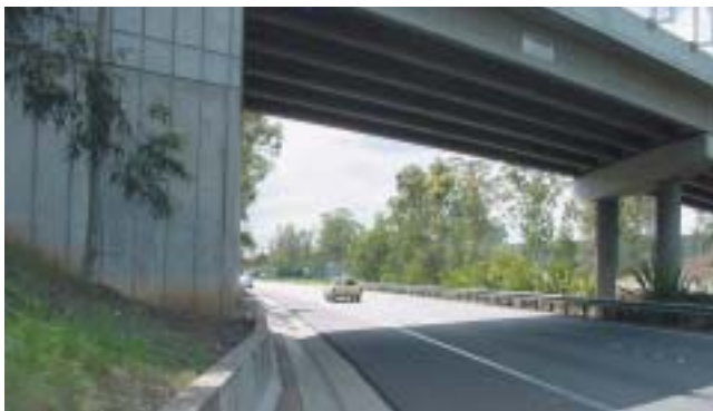
The headstock and pier combination on this bridge adds unnecessary complexity and detail.
