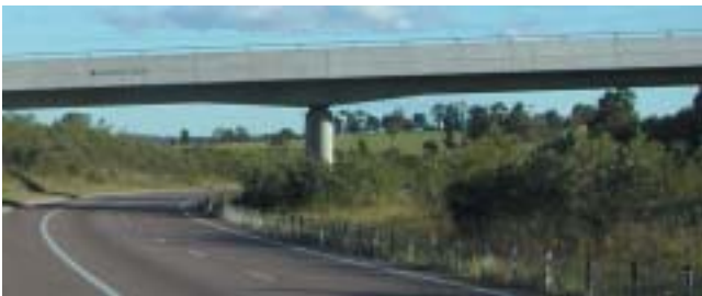
Haunched girder on bridge over the F3 Freeway at Blackhill Road, near Newcastle. The haunching is made less elegant by the abrupt angle of transition between haunched section and horizontal beam. (Also note the solid parapet and its effect on bridge slenderness).
