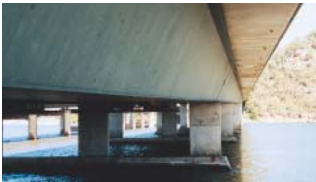
Bridge over the Hawkesbury River at Brooklyn. The angled girder increases the shadowing effect and emphasises the bridge deck and parapet.
