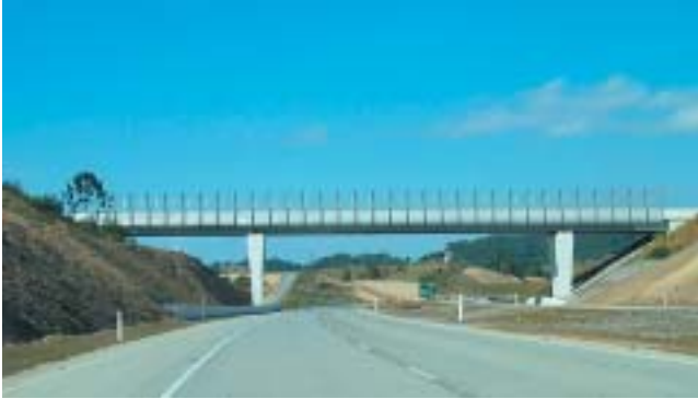
The outer spans of this bridge are not the same dimension and the symmetry of the bridge is affected.
