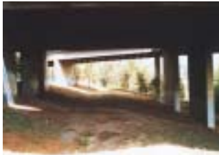
Space under bridge is undefined and erosion prone.
