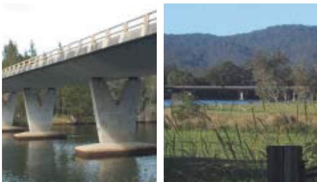
Curved soffit on the Pacific Highway bridge over the Camden Haven River near Port Macquarie.
