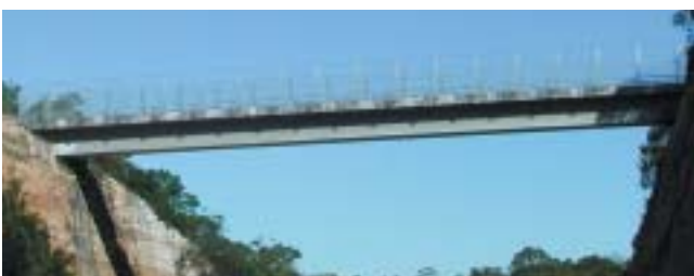
Simple single depth beam on bridge over the F3 at Cowan, NSW.
