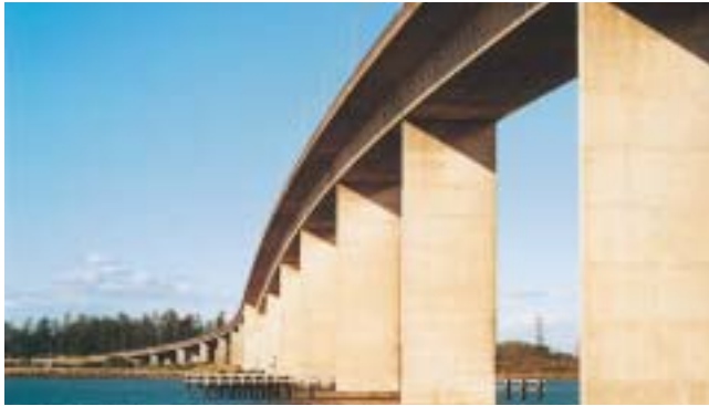
Bridge over the Hunter River at Stockton shows the effect of a right angled girder shape in afternoon sunlight.
