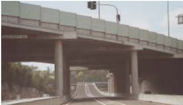
Noise walls on this bridge over the M2 significantly increase the apparent depth of the bridge, and alter the slenderness ratio.
