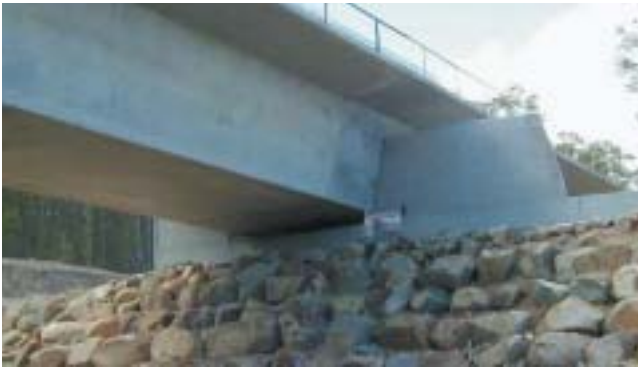
Rock abutment in contrast with the smooth concrete superstructure creates a simple and appropriate outcome. (Bridge over the Karuah River at Karuah).
