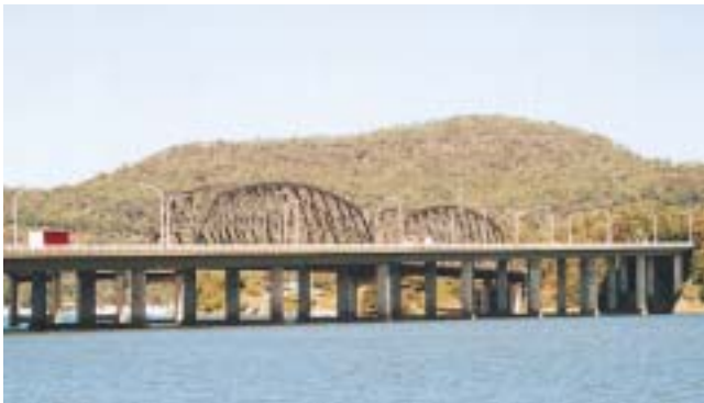
Seen from this angle there are several inconsistencies. Most notably the difference in grade and the white colorations of the barriers and lighting columns.
