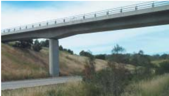
Clean, well designed rounded ends on the piers on this bridge over the Hume Highway complement the bridge and rural setting.
