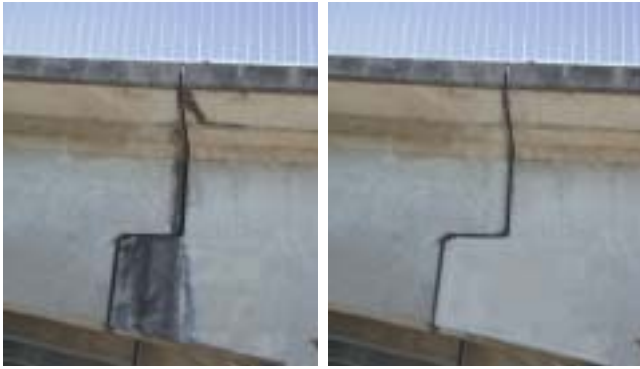
Joint detail on Fitzgerald Bridge in Raymond Terrace and photomontage of joint detail without staining. The joint is a neat simple and expressive way of supporting the girder on the piers, however staining has marred the appearance.
