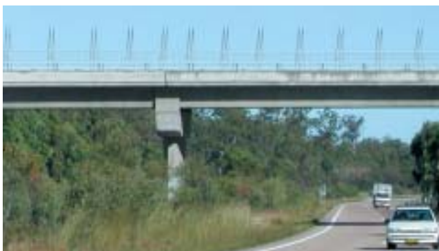
The large headstock design on this bridge over the F3 covers the gap between girders, required to accommodate mining subsidence. Its presence lacks elegance, particularly on short piers.
