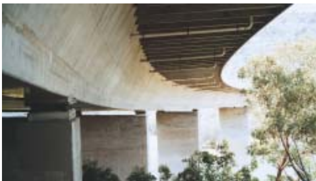
Drainage pipes on the bridge over the Woronora River hang below the outer face of the parapet.
