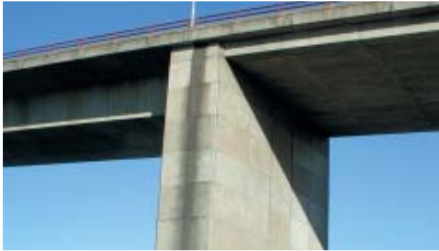
The consideration of the vertical pier to separate the varying deck depths, the recessed girders to catch the shadows, and the continuous parapet all well resolve a difficult junction.
