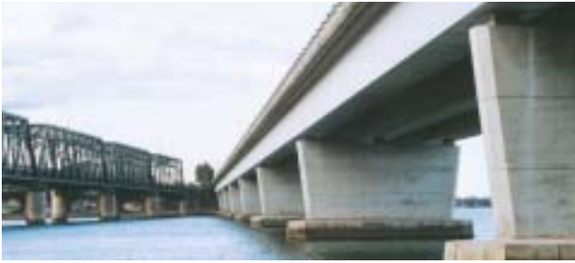
The piers on the bridge over the Georges River at Tom Uglys are reminiscent of the bow of a ship. They are well proportioned and suitably simple considering the proximity of the adjacent truss bridge. (The taper on the piers is 1 in 8).
