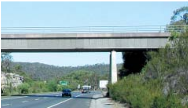
The shorter piers on this bridge over the F3 Freeway are also tapered.
