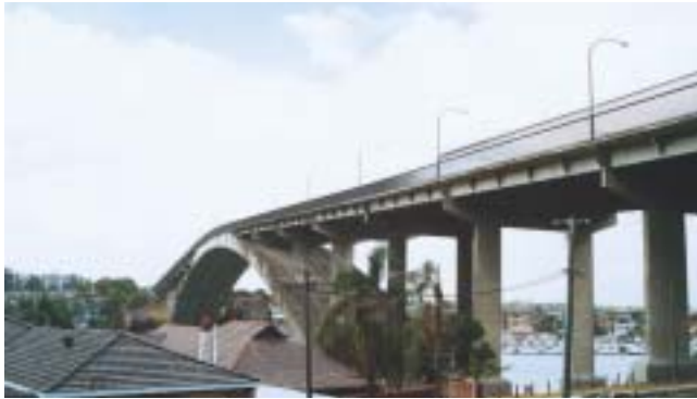
Lighting columns on the Gladesville Bridge are located and integrated with the deck support structure.
