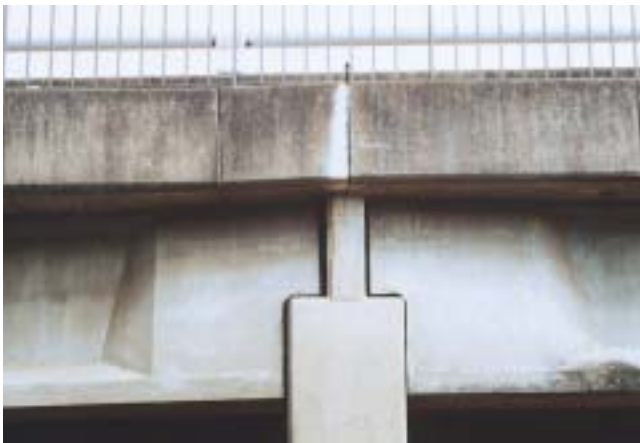
Bridge over the Tarban Creek. Recessing the pier and joint might have masked the inevitable gaps in the joint in shadow and accentuated the horizontal girder improving an otherwise well considered detail.
