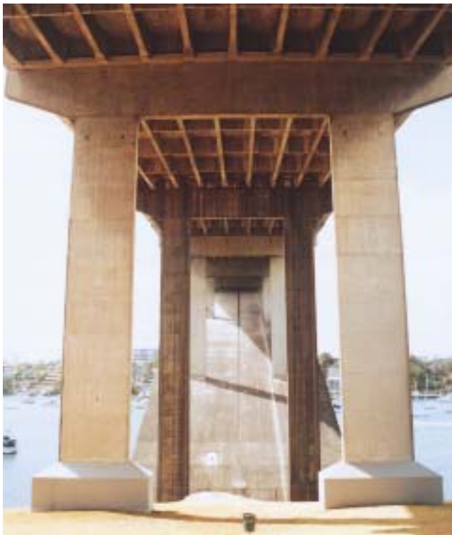
The pile caps on the Gladesville Bridge are also in keeping with the large piers providing a suitable structural termination in the park. Note the headstocks which in this context are entirely appropriate and echo the shape of the pier footing.
